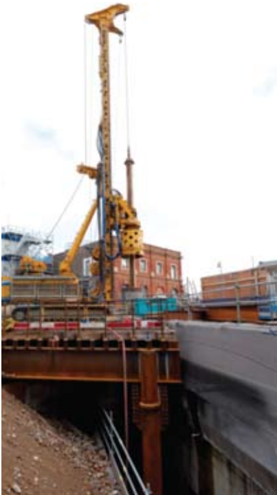
Figure 6 Suspended temporary piling platform, designed to limit piling rig surcharge on an adjacent brick-arch tunnel
